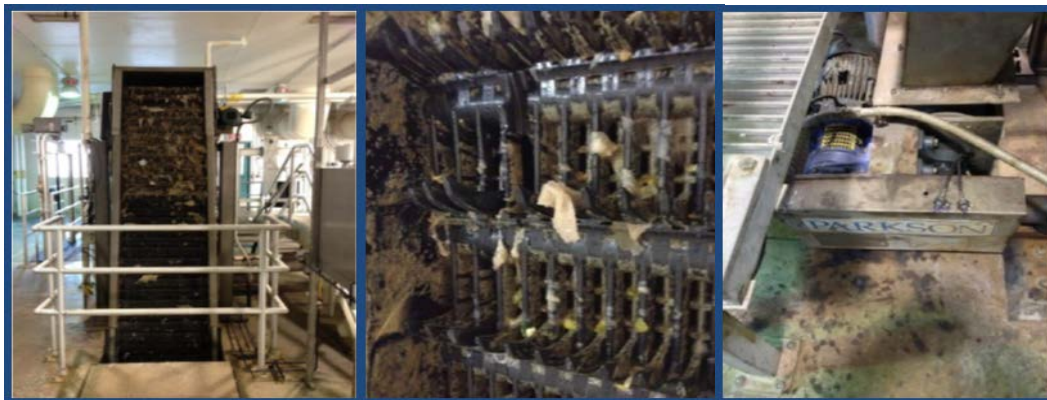
Existing Influent Screens
