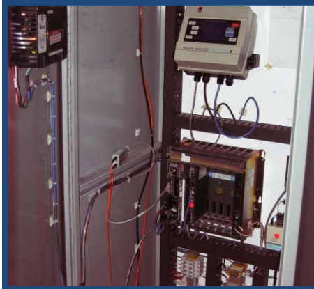
Existing PLC Installation
