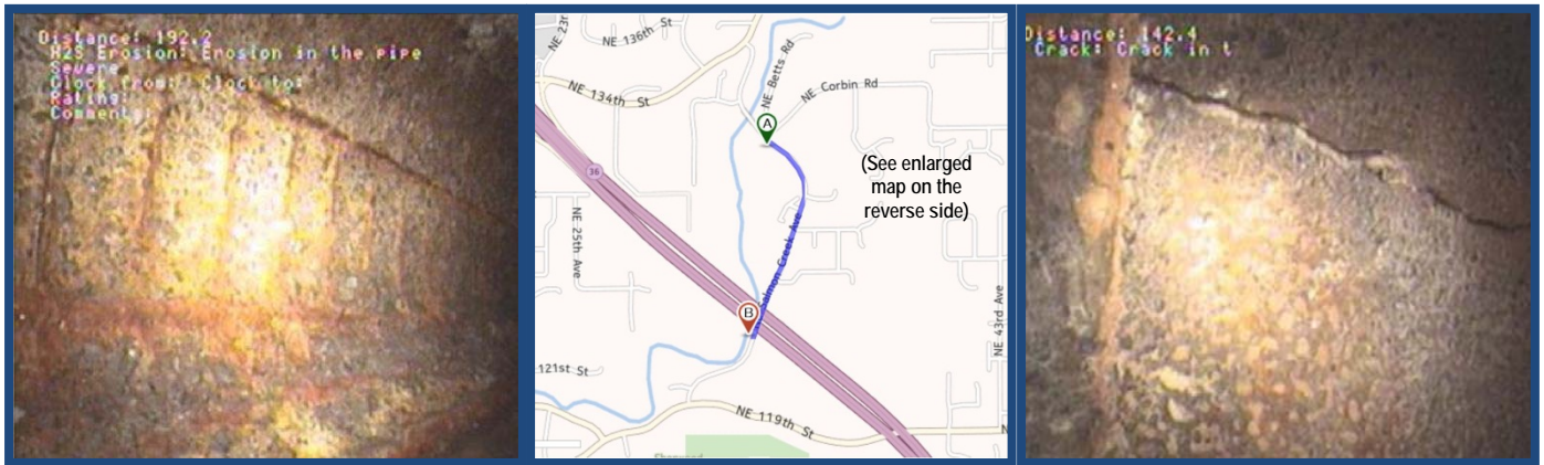
Erosion in the Pipe – Near Corbin Road
