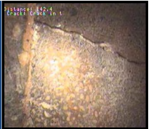
Crack in the Pipe – South of 127 th Street
