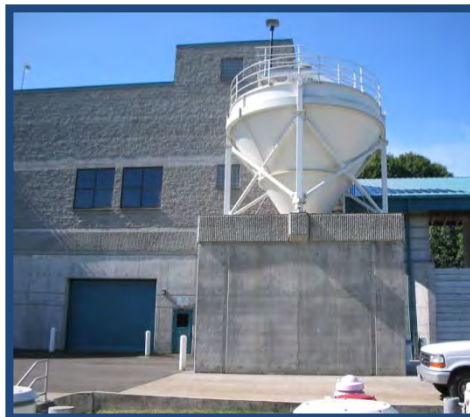
SCTP Solids Processing Center
