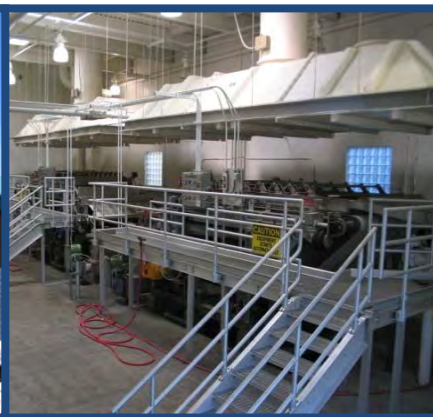
Existing Sctp Belt Filter Press
