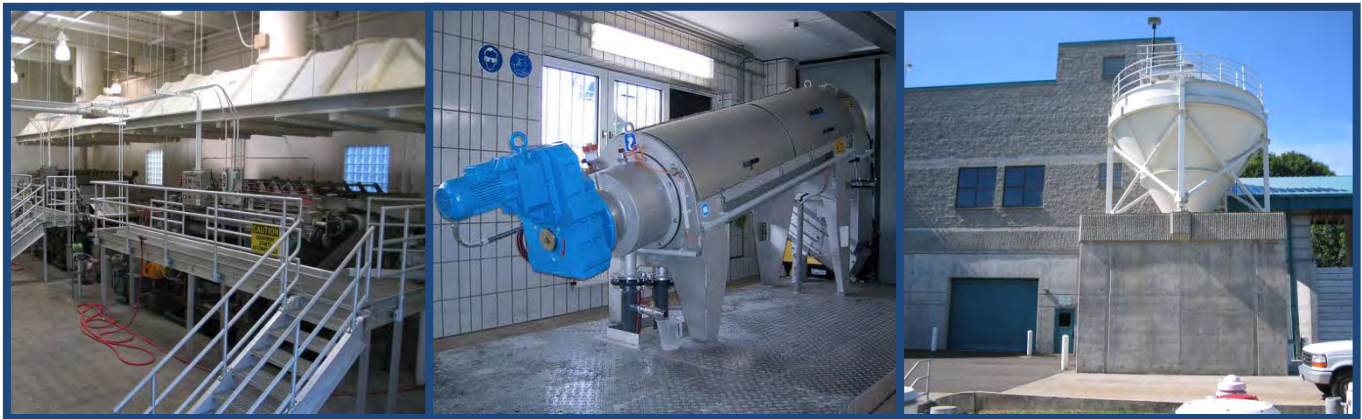
Existing SCTP Belt Filter Press
