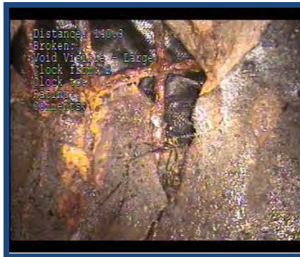
Signs of Failure of the Interceptor
