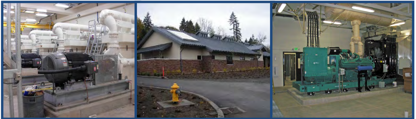
Existing Pump Assembly
