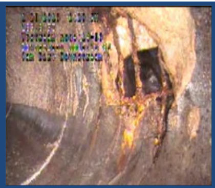
Rebar Showing at Failure Location
