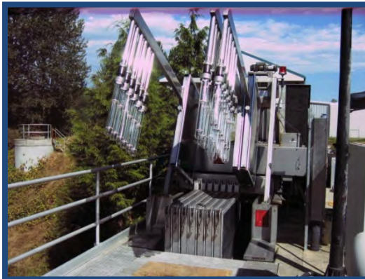
Existing UV System
