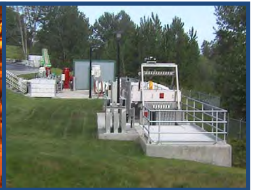
Existing UV Disinfection
