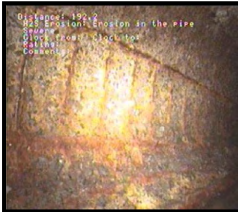
Erosion in the Pipe – Near Corbin Road
