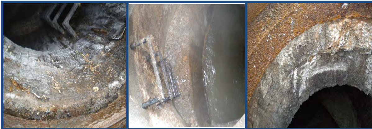
Corrosion Around Manhole Rim
