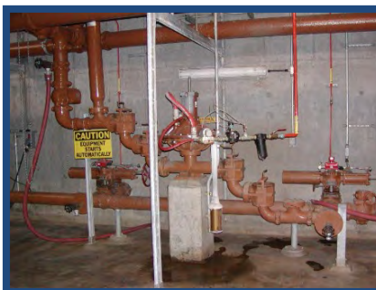
Existing Diaphragm Style Pump
