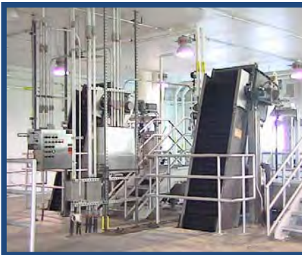
Existing Influent Screen
