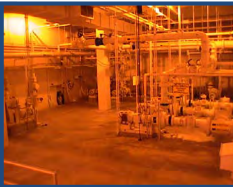
Existing RAS/WAS Pump Station
