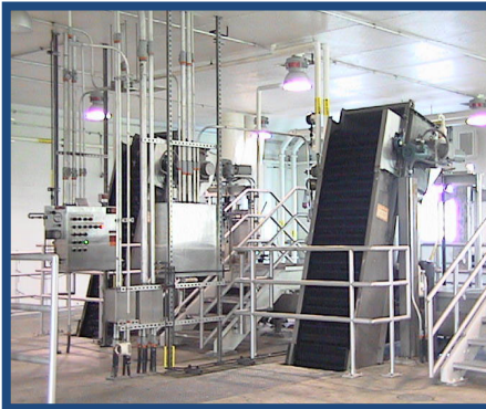
Existing Influent Screen
