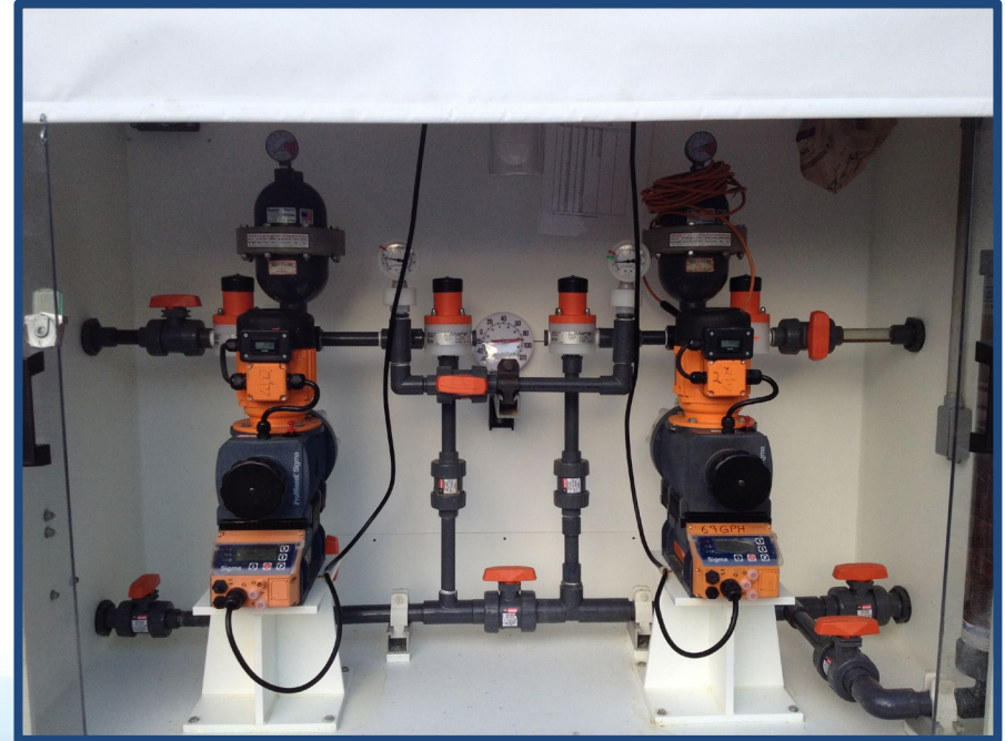
Example Chemical Dosing Setup
