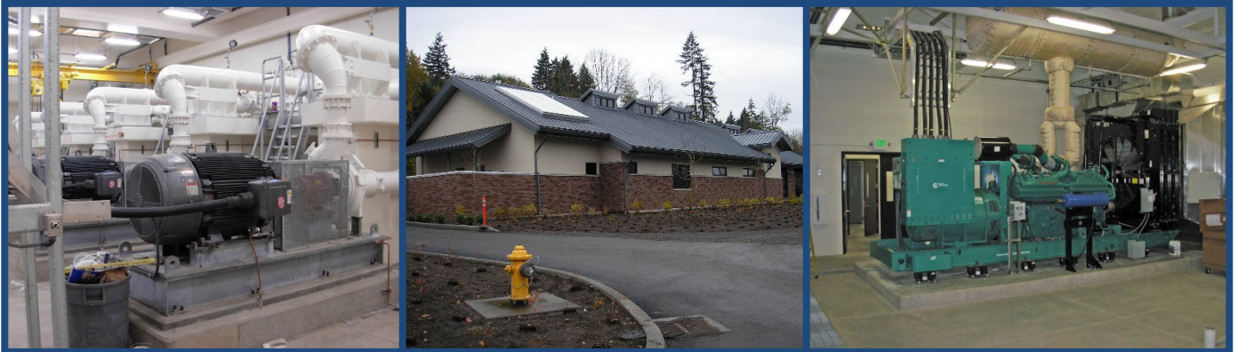
Existing Pump Assembly
