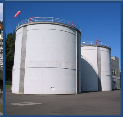
Existing Anaerobic Digester
