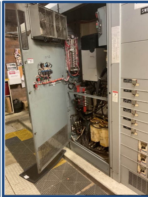
Existing VFD cabinet and harmonic filter
