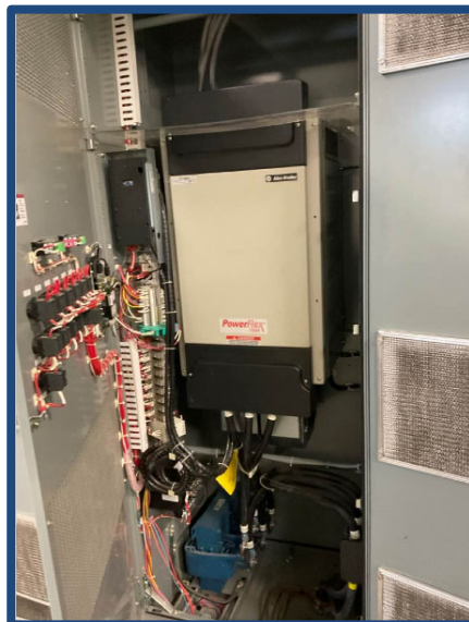
Existing 117 th St Pump Station VFD Cabinet
