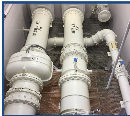
New Influent Flow Meters
