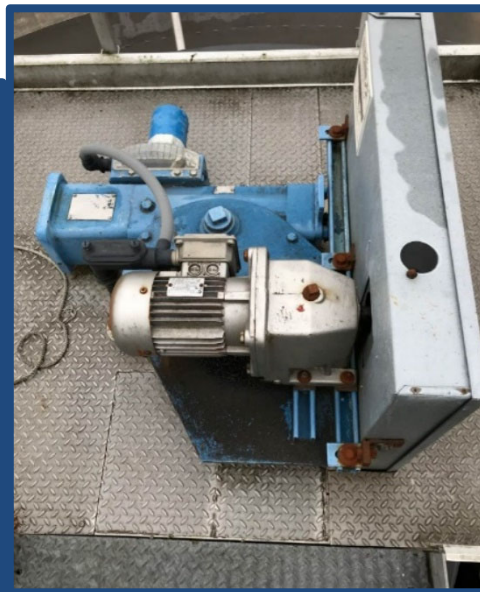
Existing Clarifier Motor and Drive
