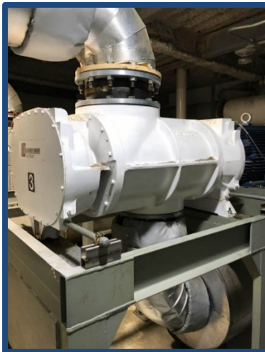
Existing Positive Displacement Blower
