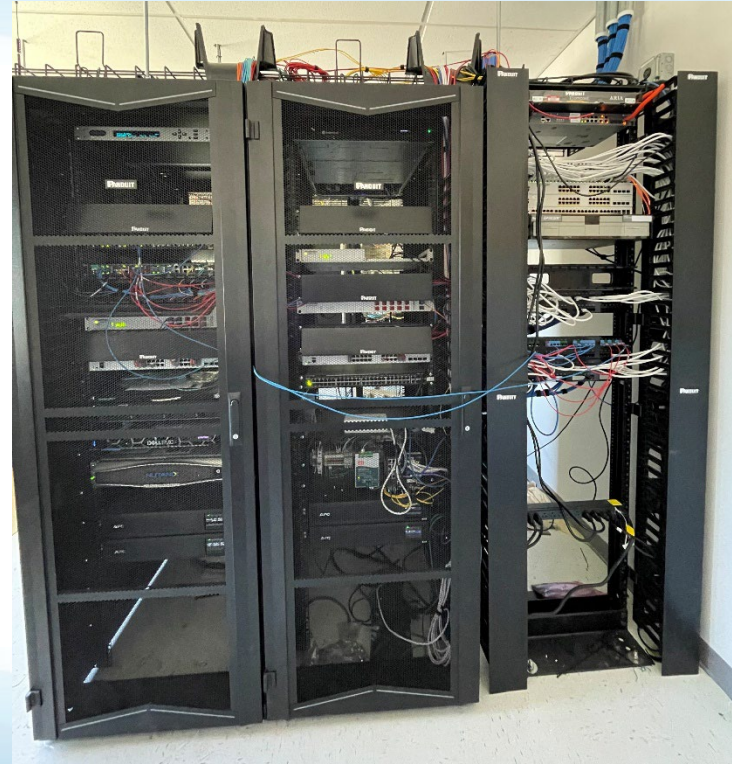
New Server Cabinet
