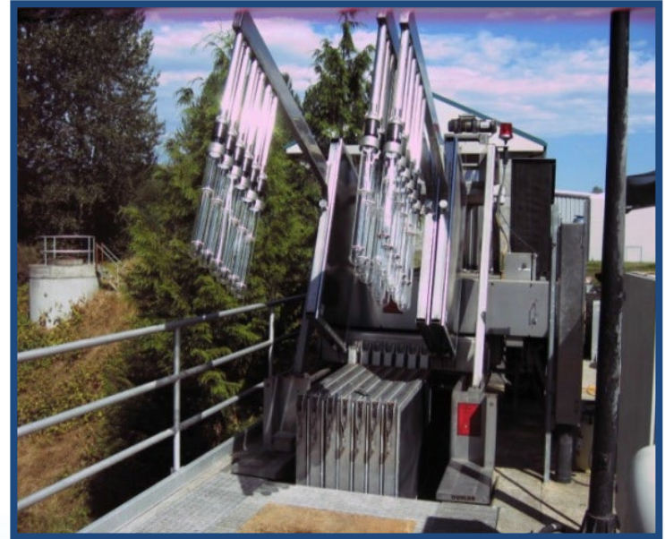
Ultraviolet (UV) System
