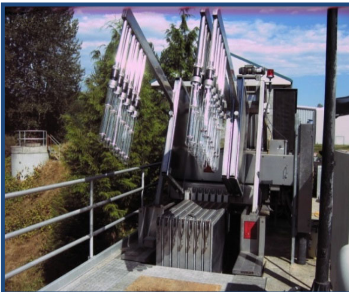
Existing UV System
