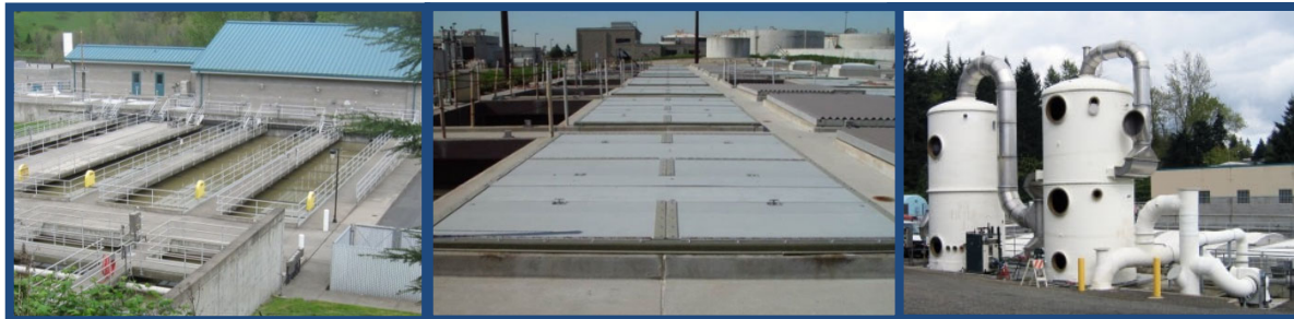
Existing Primary Clarifiers
