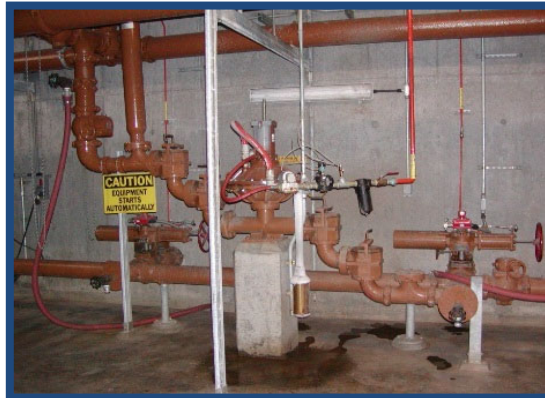
Existing Diaphragm Style Pump
