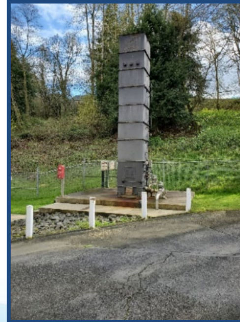
Defunct Waste Gas Burner
