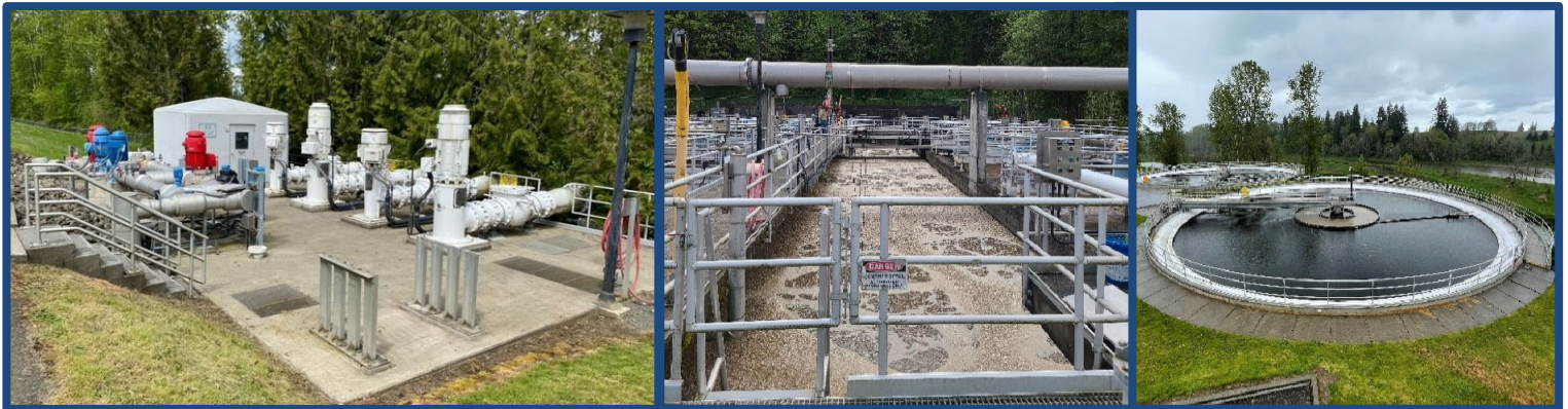
Existing Effluent Pump Station
