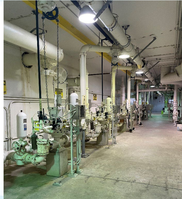
Primary Sludge Pump Gallery
