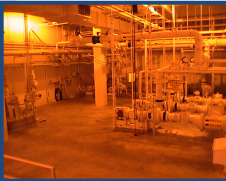
Existing RAS/WAS Pump Station
