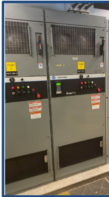
Existing VFD cabinets
