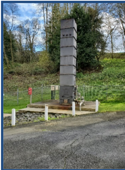
Defunct Waste Gas Incinerator (Sur-lite)
