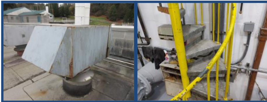
SCTP Corroded Supply Fan
