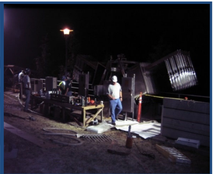
Existing UV System Expansion During Phase 4
