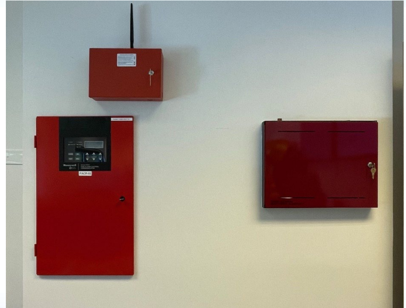
New Fire Alarm Panel
