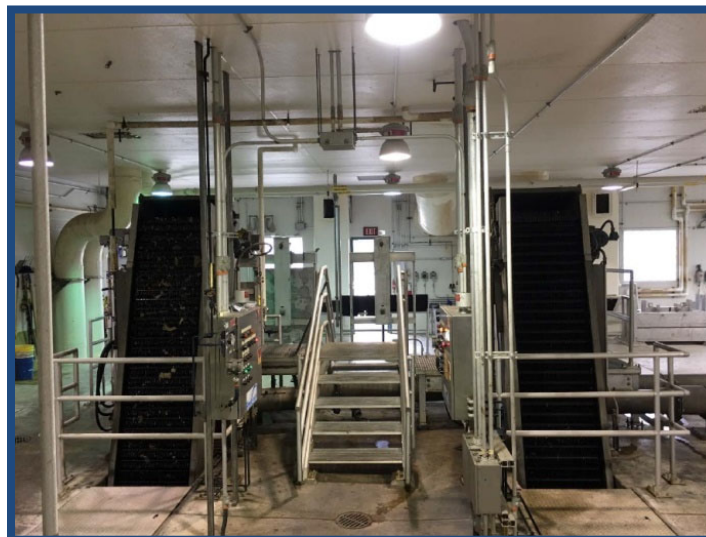
Existing Influent Screens Rebuilt in 2017
