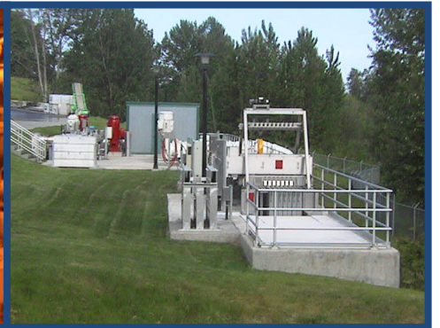
Existing UV Disinfection
