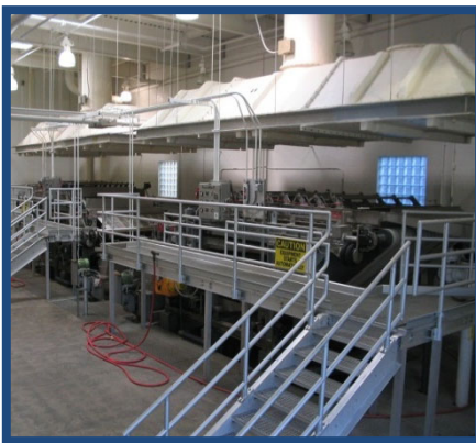
Existing Sctp Belt Filter Press
