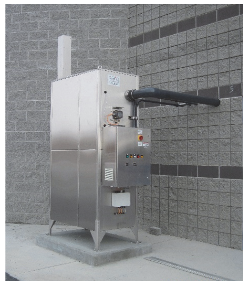
Figure 3-6. Photoionization Unit (90 cfm) Orem Utah
