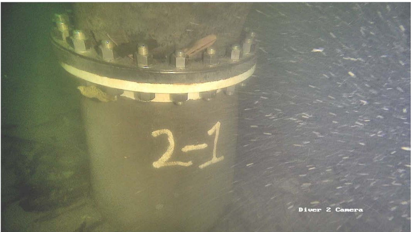
Figure 5 - Diffuser #7 riser pipe.
