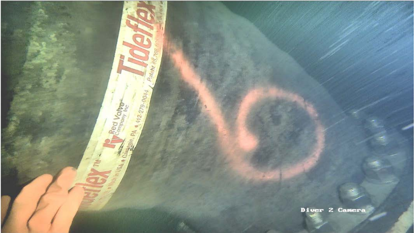
Figure 6 - #6 diffuser check valve.
