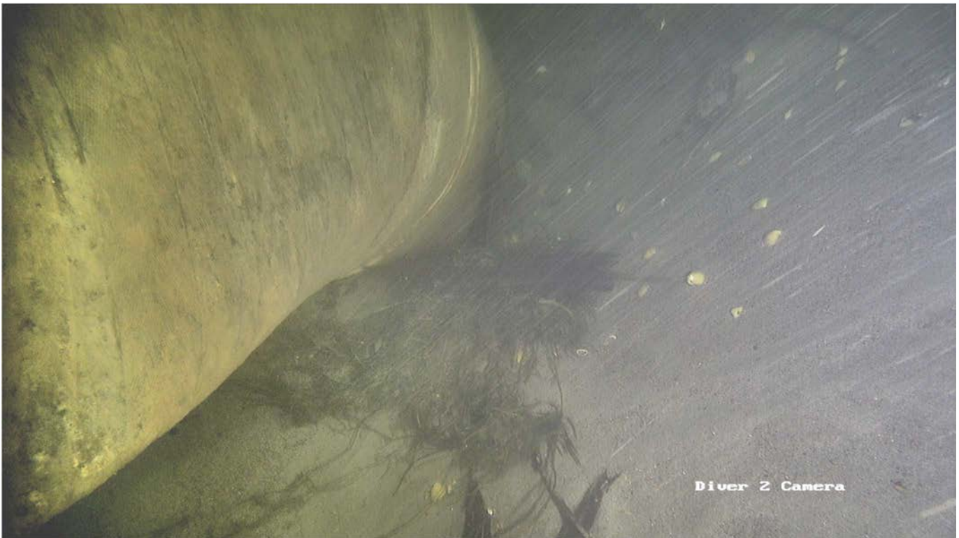
Figure 7 - Light wood debris accumulation on some diffusers.
