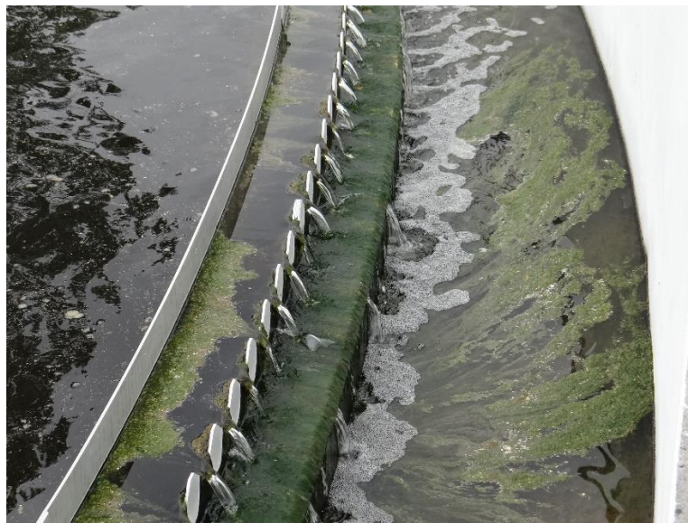
Picture 4-5: Algae in Secondary Clarifiers
