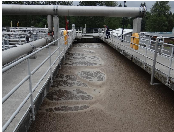
Picture 4-2: Aeration Basins
