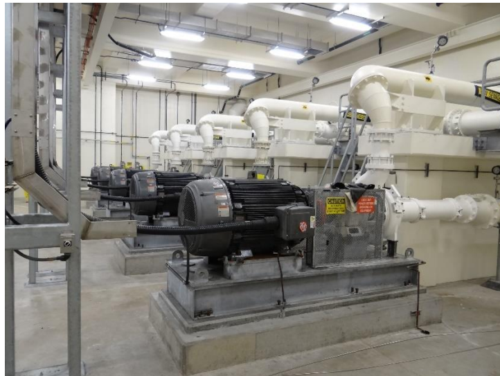
Picture 4-12: 117 th Street Pump Station Pump Room
