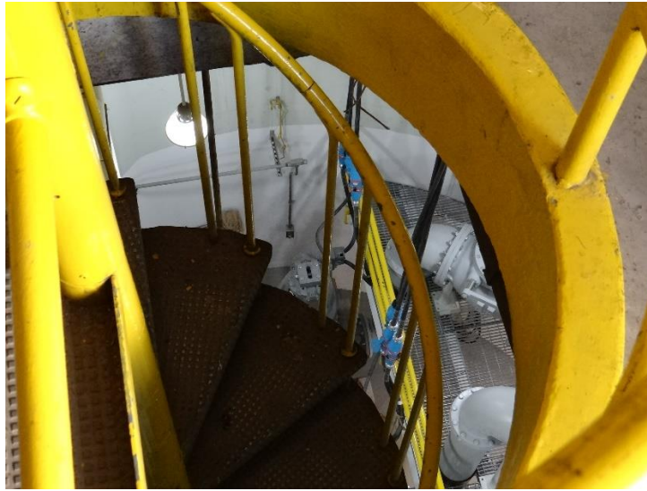
Picture 4-11: 36 th Avenue Pump Station Dry Well
