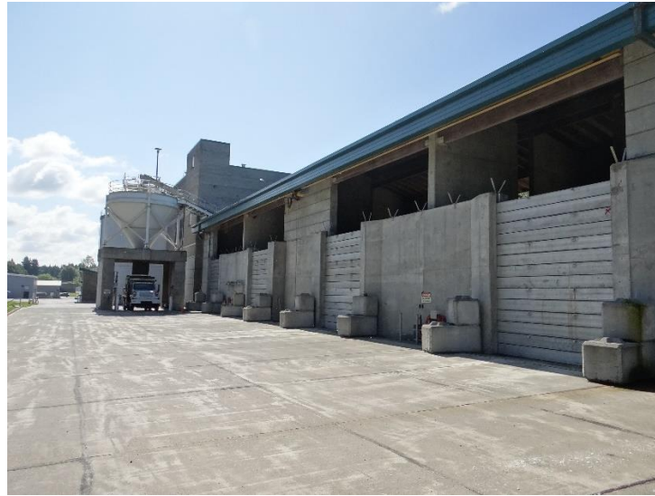
Picture 4-3: Sludge Drying Beds
